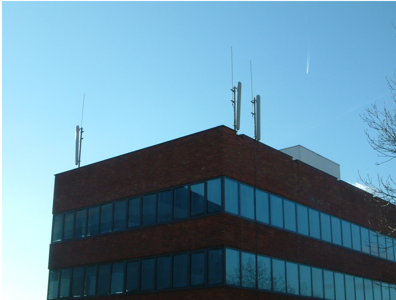
Picture 4.1 Rooftop masts such as these do not generally need the Council's permission
